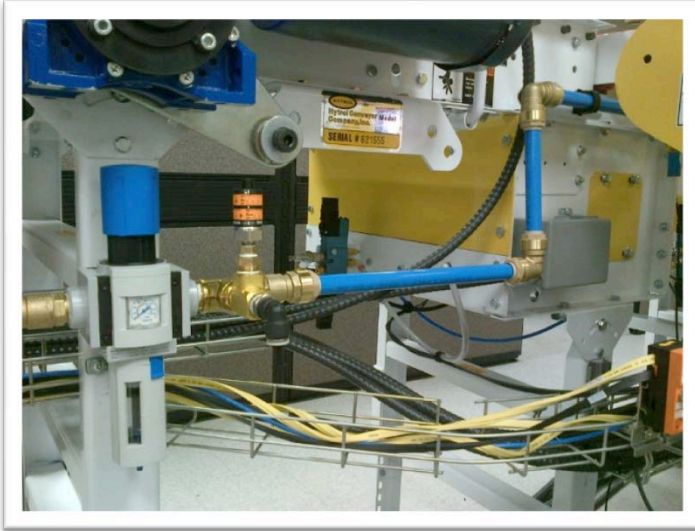
Pneumatic air supply with pressure sensor. Used to alert system to low air pressure.
