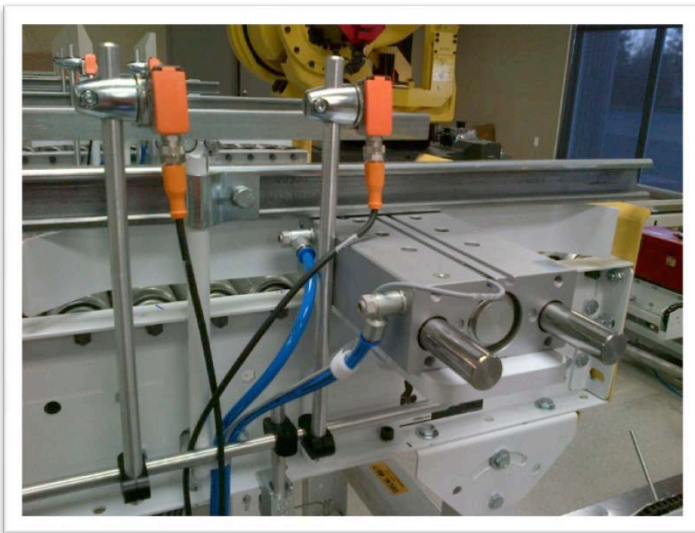
Case pusher cylinder with case presence proximity switches. Case pushers adjustable design for case change overs. Sensor bracketry allows for easy movement of sensors.
